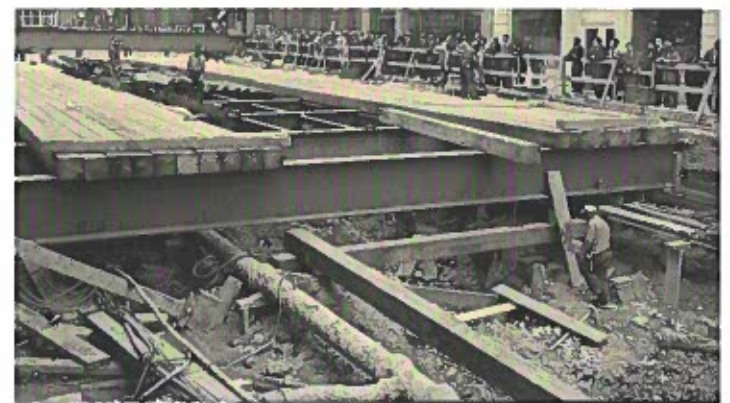
Toronto's subway line provided some commuters with an alternative. Here, Yonge Street is planked to allow traffic on top of the construction.
