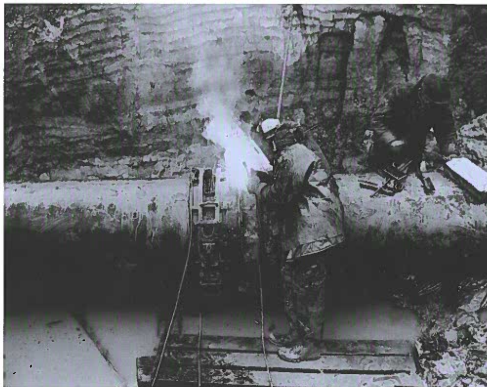
The final weld on the Trans-Canada pipeline was made at Kapuskasing, Ontario, October 1958.
