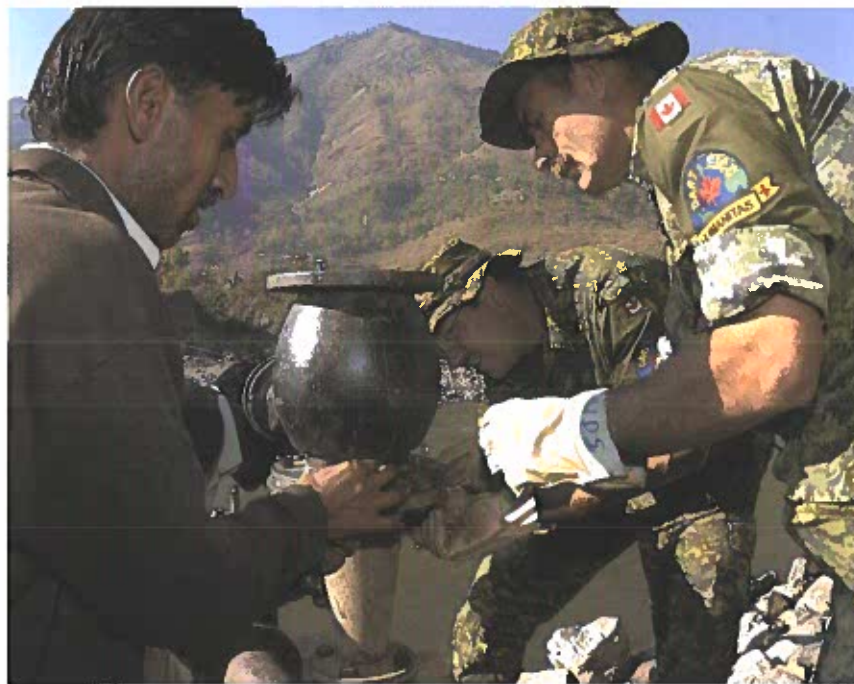
Construction engineers with the Canadian Forces Disaster Assistance Response Team help villagers in Pakistan rebuild a water pump after the 2005 earthquake. The engineers are helping villagers restore the vital water supply.
